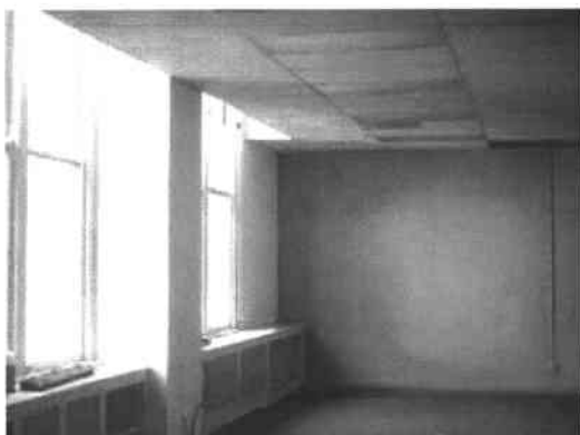
The dropped ceilings covering an air conditioning system also cover the historic windows, altering their proportion and resulting in loss of the historic character. Photo: NPS files.
