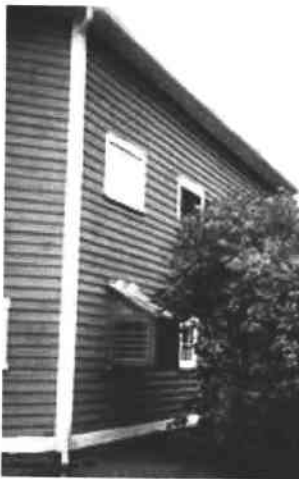
Installing a fan (successfully concealed here) for increased ventilation can be a successful low-tech substitute for air conditioning. Photo: Courtesy, Shelburne Village.
