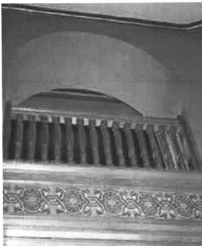
A return air grille is successfully screened behind the arch. Photo: NPS files.
