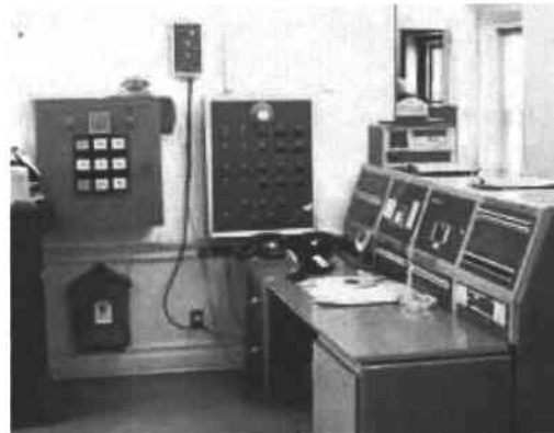
Complex mechanical systems for institutional buildings may require a central control room. Photo: NPS files.
